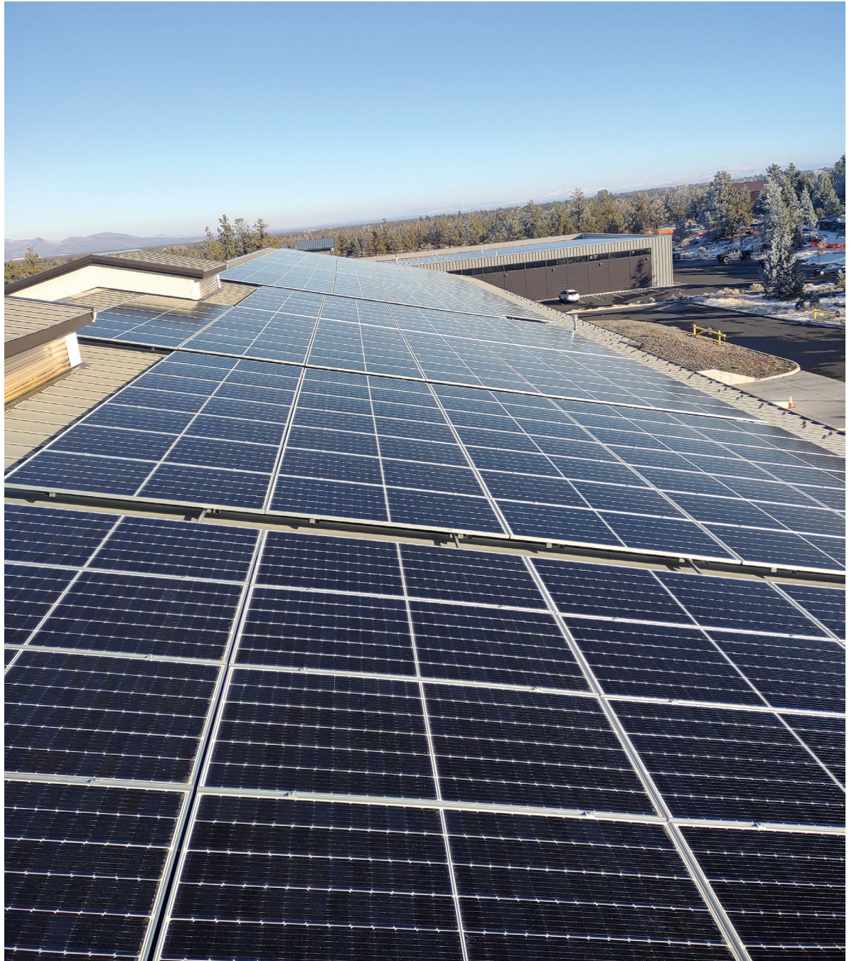
PHOTO | COURTESY SUNLIGHT SOLAR
