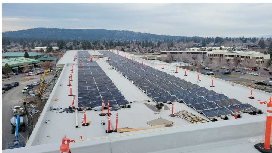
THE CURRENT'S SOLAR ARRAY WILL GENERATE ENOUGH ENERGY TO POWER 100% OF THE BUILDING'S LIGHTING, COOLING, ELEVATORS AND VENTILATION | PHOTO COURTESY SĀJ ARCHITECTURE
