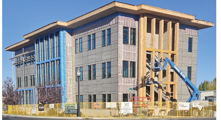
LCHC'S THREE-STORY WELLNESS CENTER IS SLATED FOR COMPLETION IN SPRING 2025 | PHOTO BY ANDREA HINE
