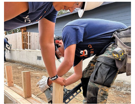
YOUTHBUILD PARTICIPANTS BUILD FORMS FOR THE FOUNDATION AT THE SISTERS HABITAT BUILD SITE | PHOTO COURTESY OF YOUTHBUILD
