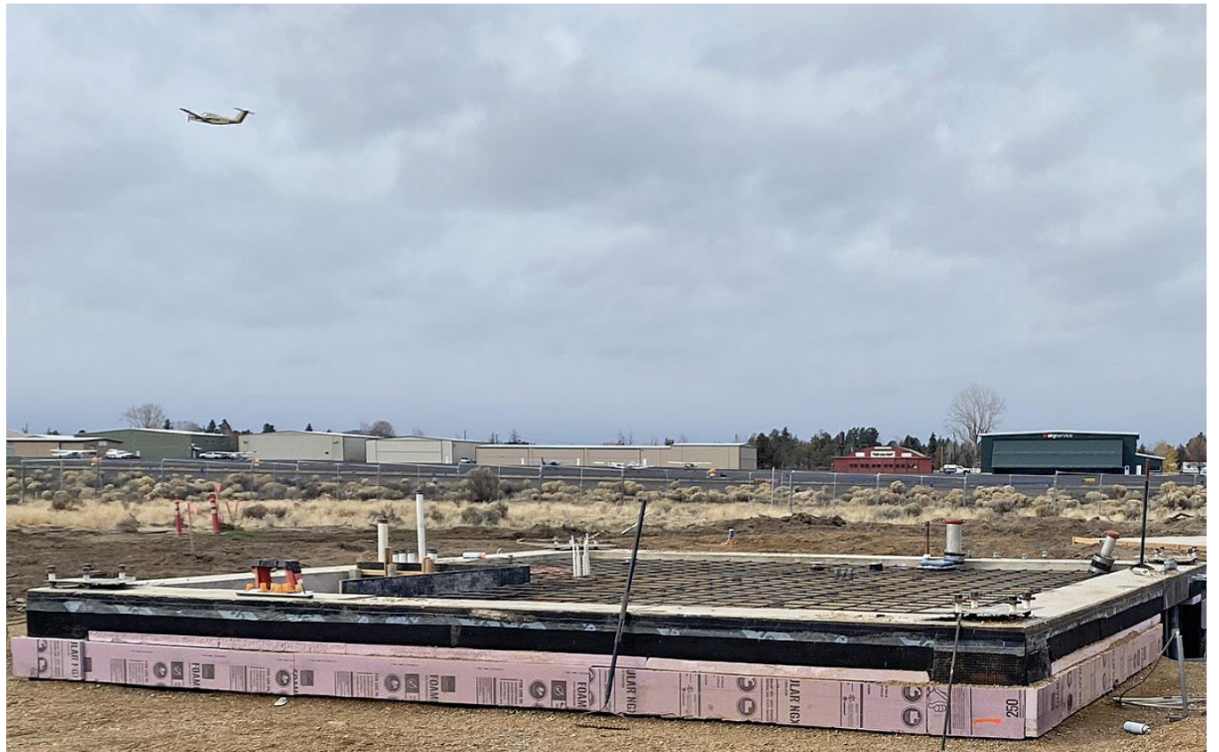
THIS "BEFORE" PHOTO SHOWS THE CONTROL TOWER DURING ITS FIRST STEPS OF CONSTRUCTION | PHOTO COURTESY OF MORRISON-MAIERLE
