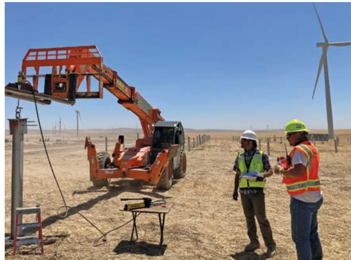
IAIN SMITH OF CTI ON SITE TESTING AT A SOLAR FARM PROJECT
