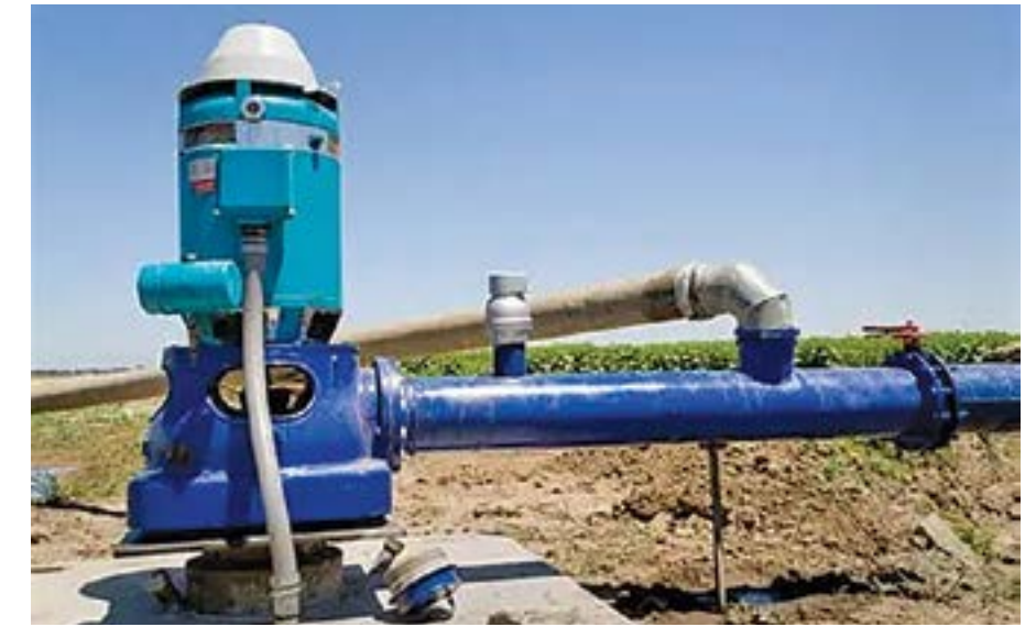
STETTLER SUPPLY HAS FOUND THAT IMPROVEMENTS IN TECHNOLOGY HAVE MADE WATER MANAGEMENT EASIER. (PHOTO COURTESY OF STETTLER SUPPLY COMPANY)
