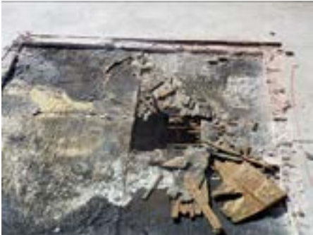
DAMAGED ROOF SHEATHING CAUSED BY INADEQUATE INSULATION
