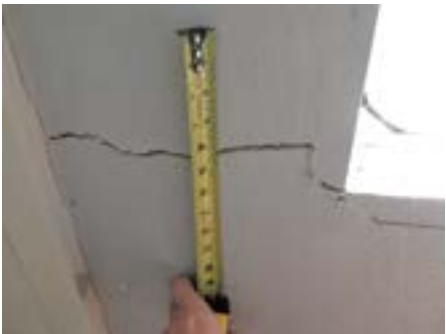
DRYWALL CRACK AT WINDOW CORNER CAUSED BY FOUNDATION MOVEMENT
