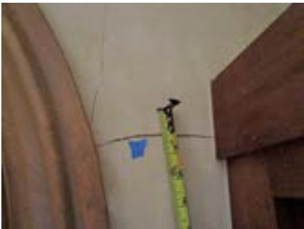
INTERIOR FINISH DAMAGE CAUSED BY FOUNDATION MOVEMENT
