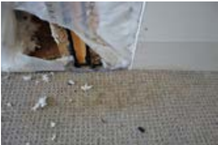
WINDOW WATER LEAKS RESULTED IN DAMAGE TO DRYWALL AND CARPET | PHOTOS COURTESY OF ASHLEY & VANCE ENGINEERING
